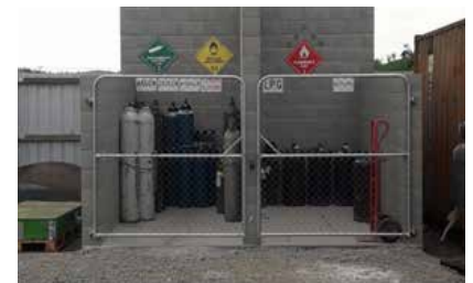
New gas storage bunker separating different classes of gases.
